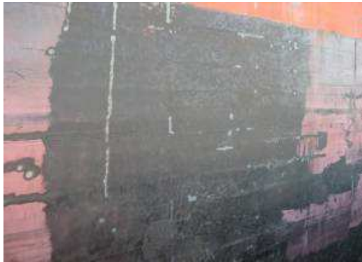
Loose paint film (Partial blast cleaning)
