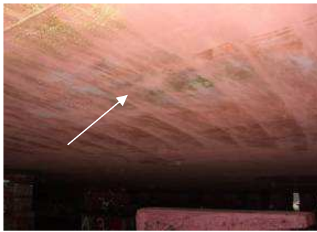
Slime layer is remained due to lack of washing down.
